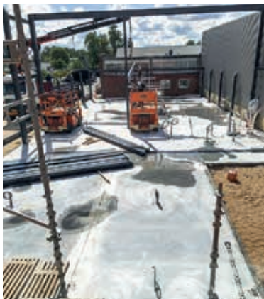
First step: an extra office block was built to connect the two existing buildings.
