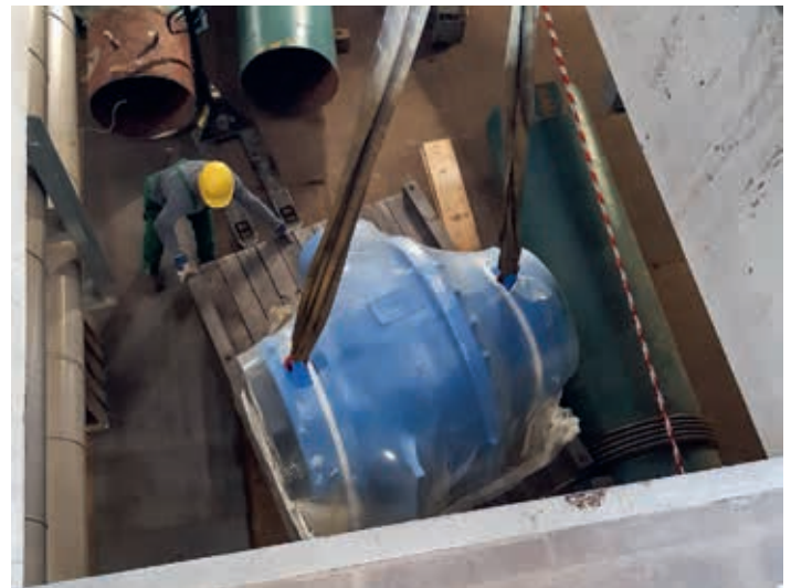
Delivering a new KHSVI ball valve from KFC to Wien Energie
